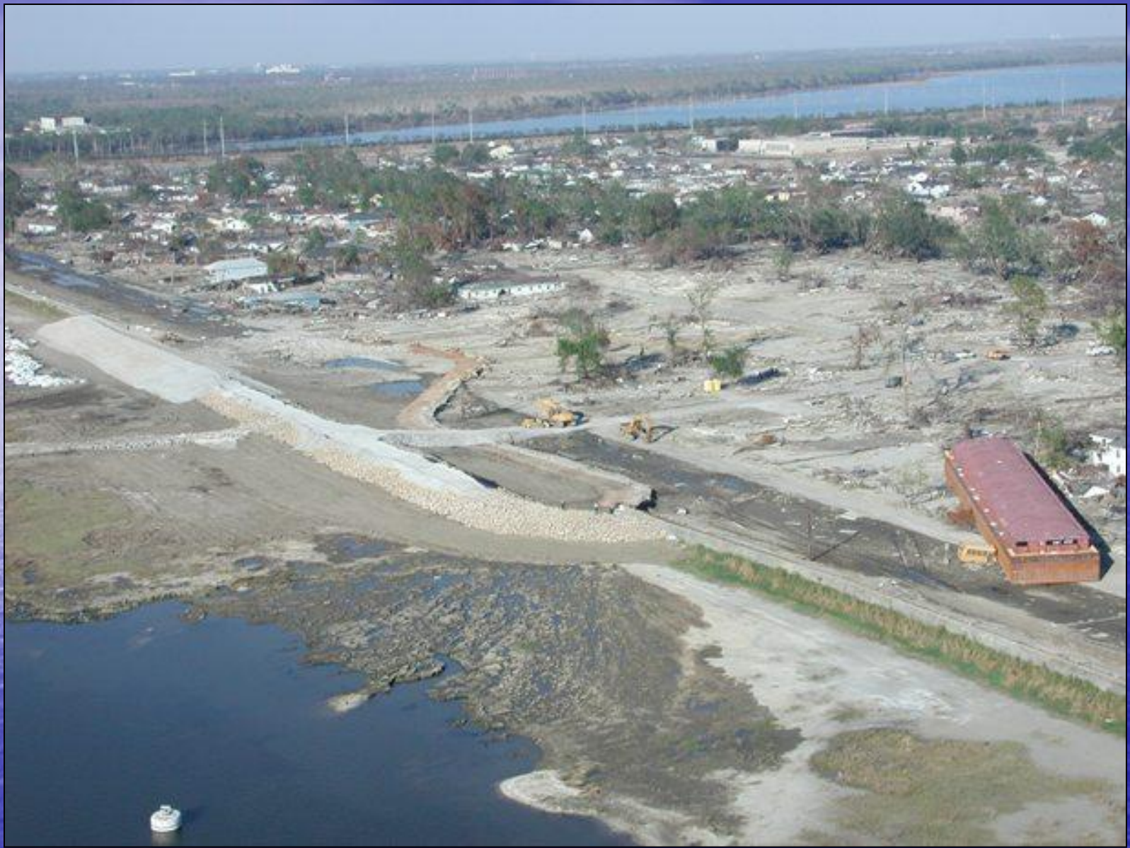
Seepage crevasse exposed at the east levee of the IHNC breach after Hurricanes Katrina and Rita
